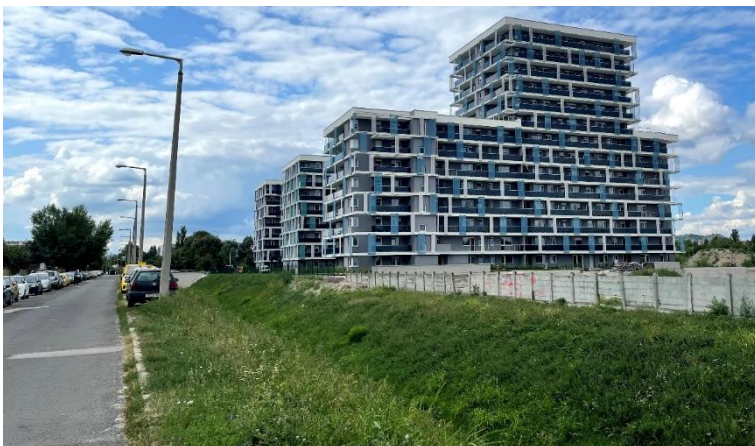
Figure 14 : Budai Walzer under construction view from the side street Source: The Author (August 2021)
