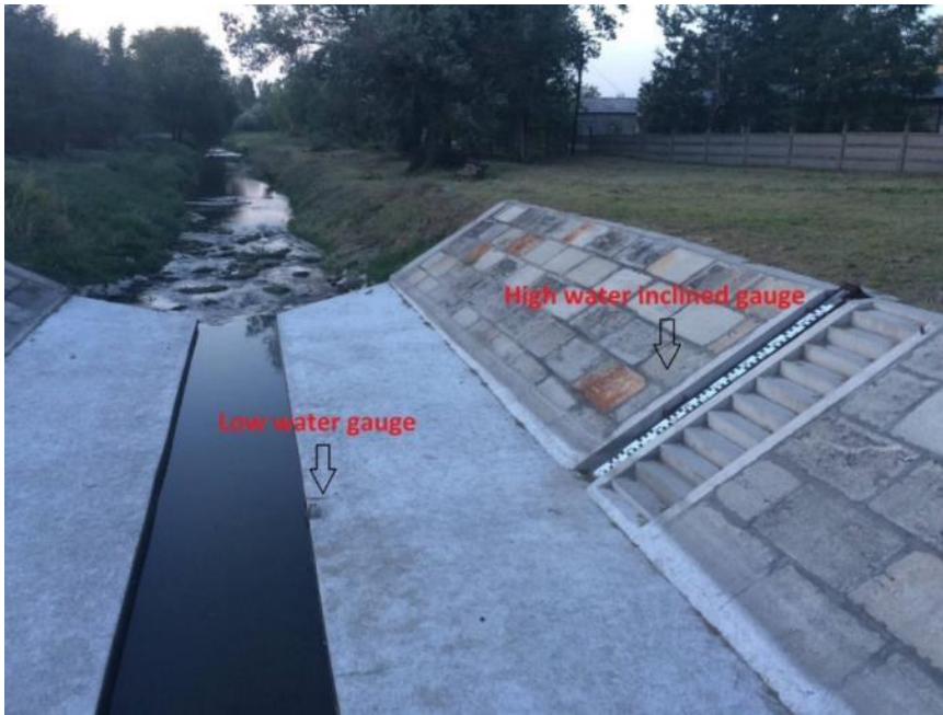
Figure 40. Low water and high water gauge
