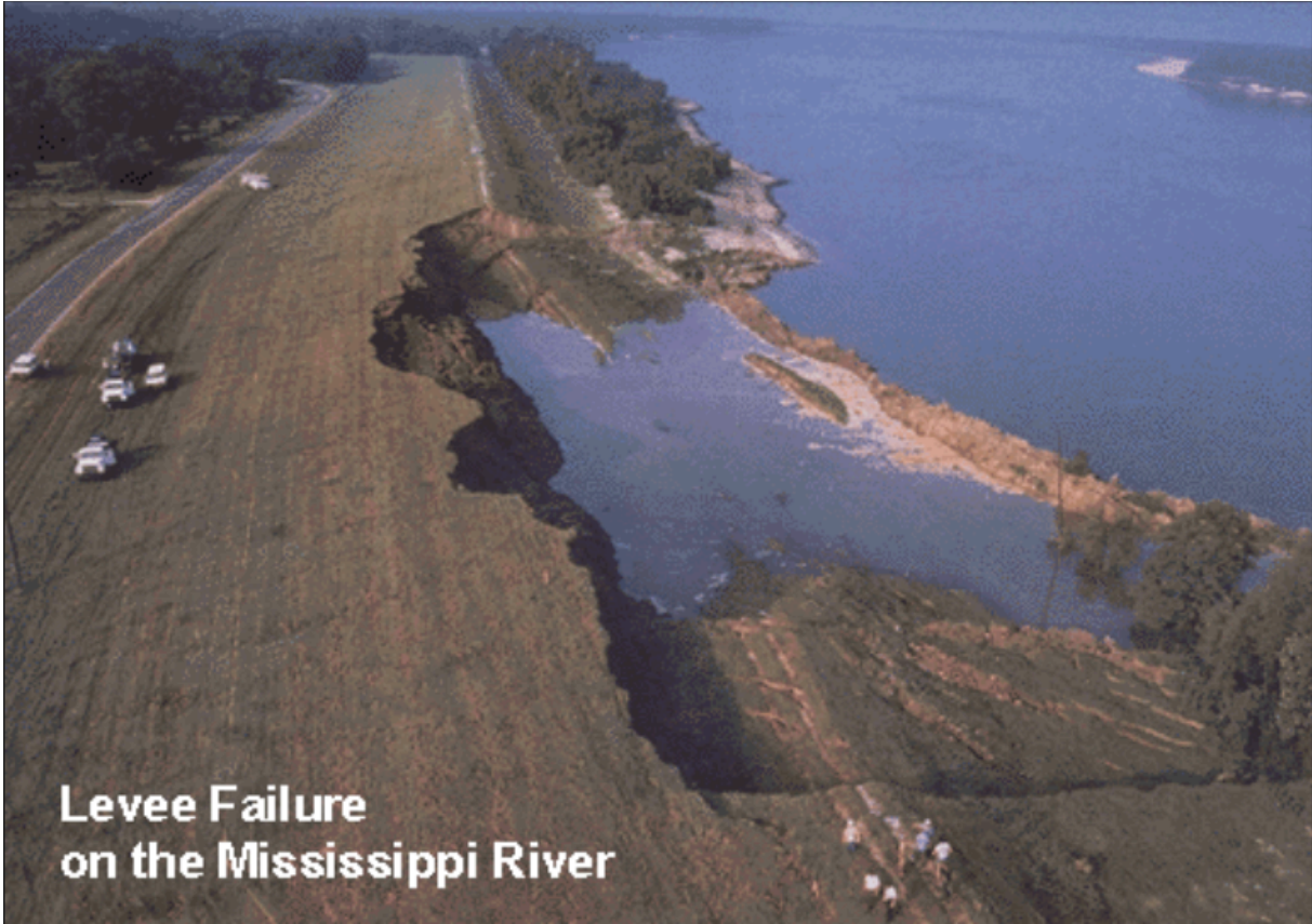
Fig. 46.: Levee failure on the Mississippi River during the 1993 flood event. [17]
